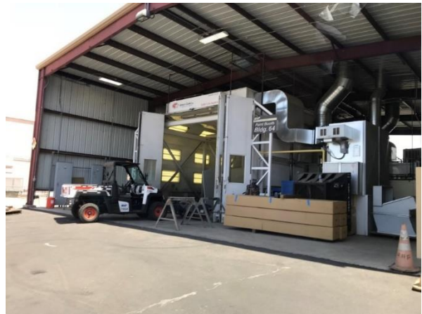
Example: Crosscut Paint Booth
