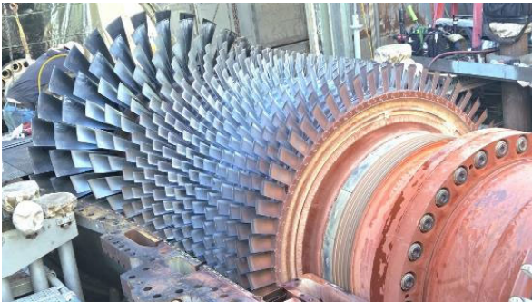
Gas turbine downstream
