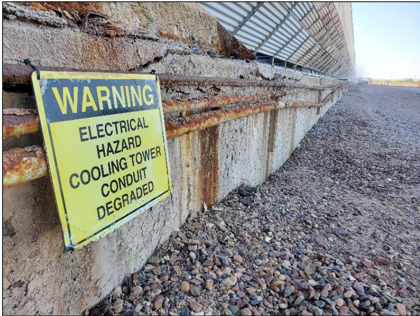
Gila River Power Station; April 2025
