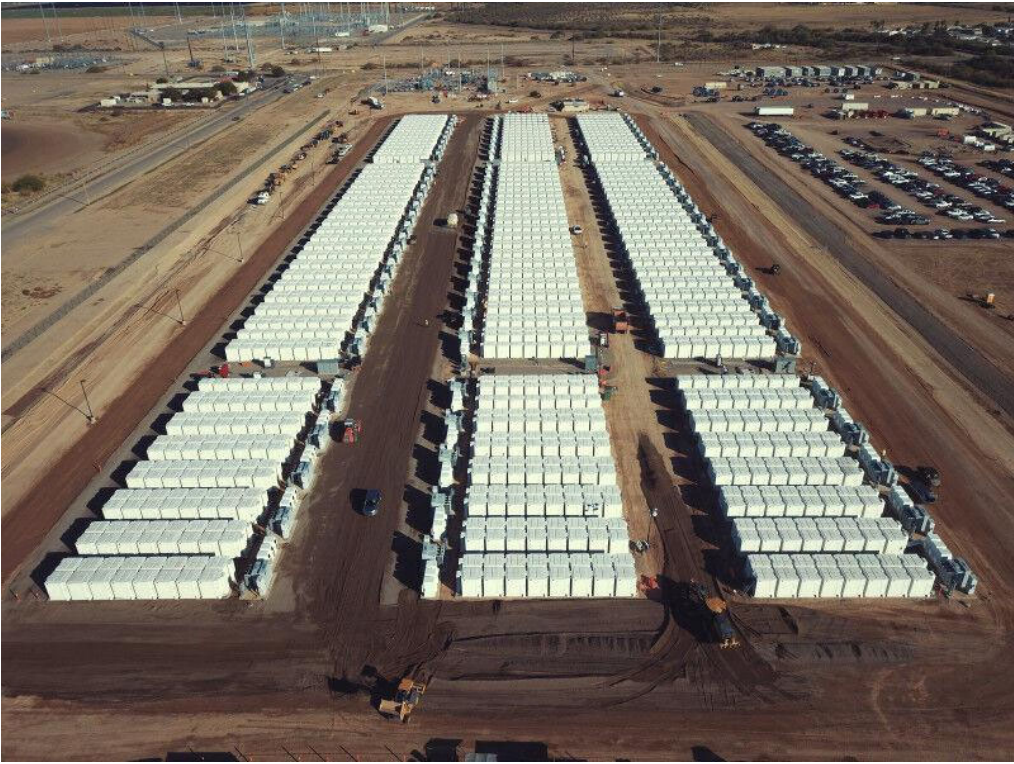
300 MW Battery Storage
