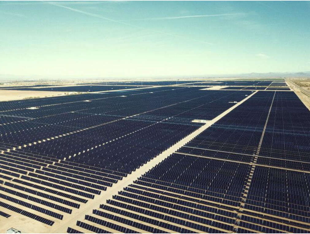
300 MW Solar Farm
