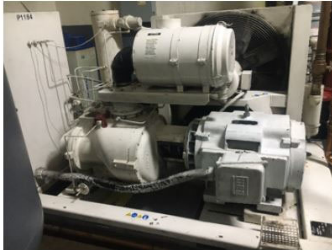
Gardner-Denver 100 HP Compressor
