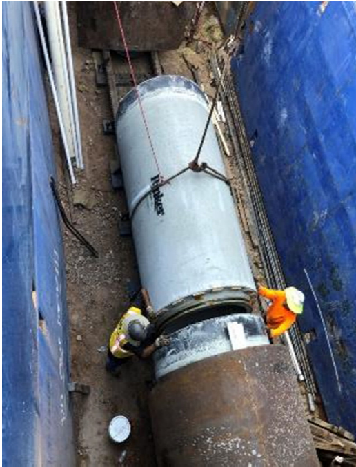
Concrete Carrier Pipe
