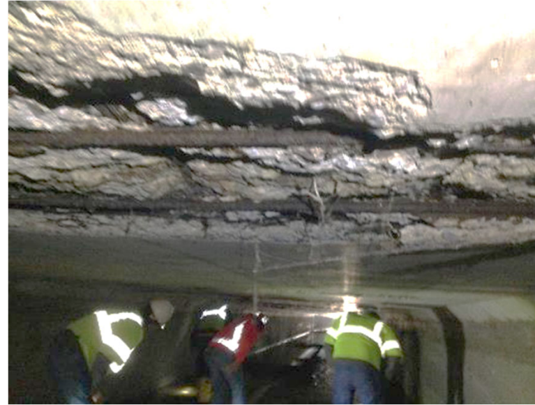
Exposed Rebar on Ceiling Wall
